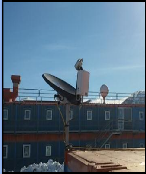
Metek MRR - Radar
