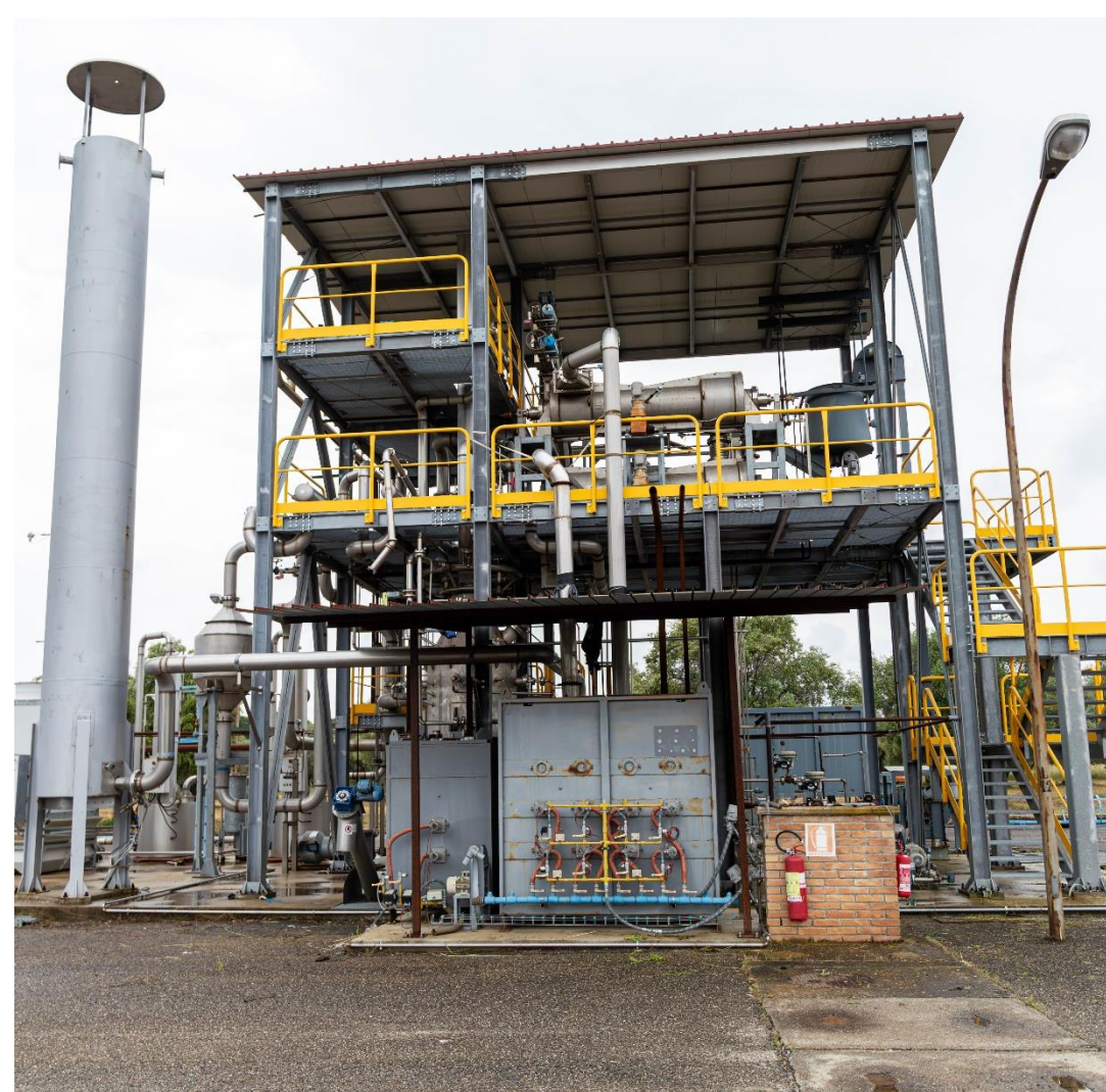
Three stage gasifier
